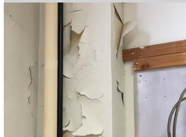
Report building damage to CPFM!
