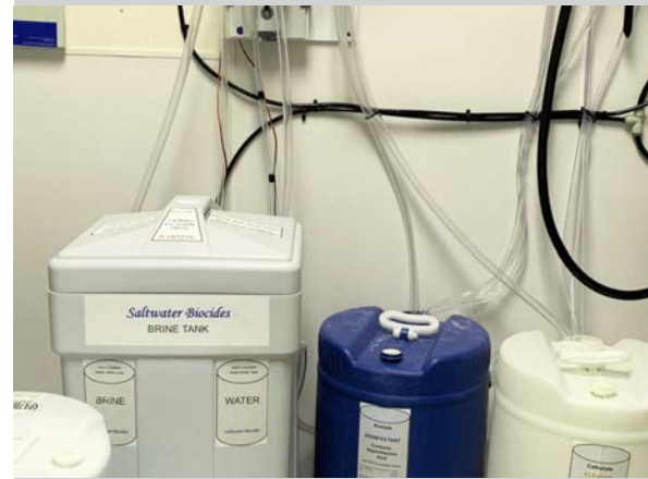
Saltwater biocide system.
