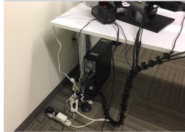
Surge protectors must plug into wall outlets, not other surge protectors!
