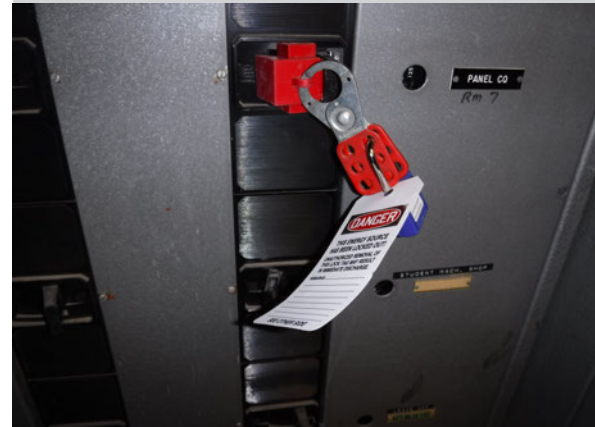
Turn off malfunctioning equipment!
