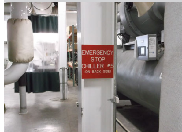
Remember electricity is not the only form of hazardous energy!
