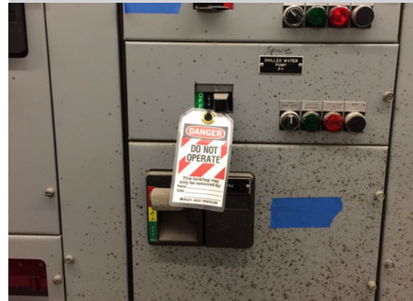
Lockout / tagout equipment before repair, or maintenance!
