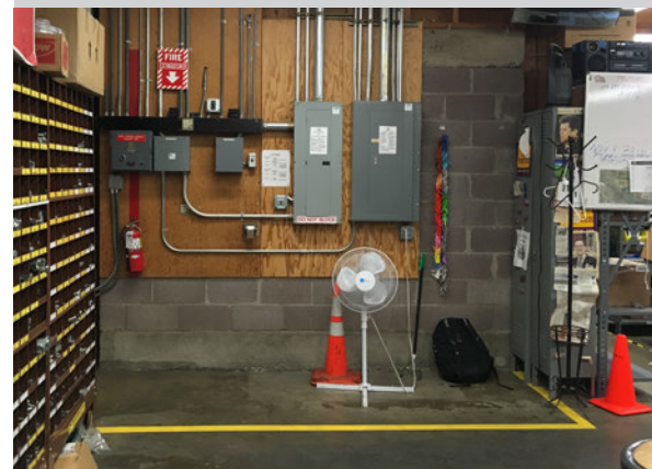
Keep electrical panels clear and closed!
