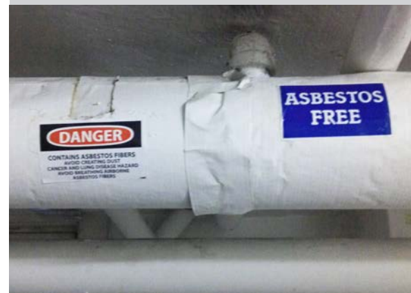
Example pipe labels for OSHA compliance and employee awareness.
