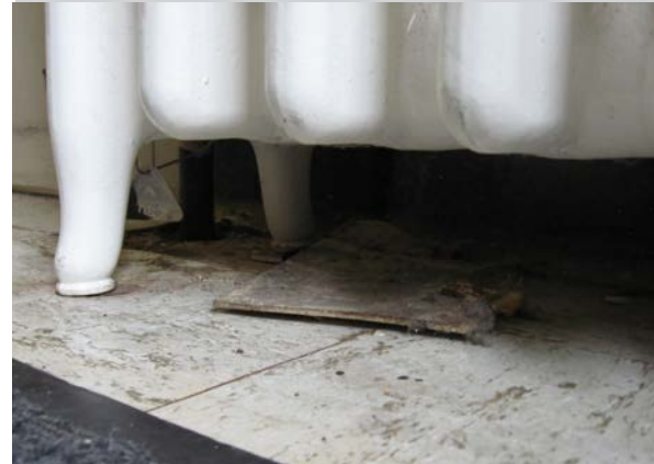
Report any damage of UO property to CPFM customer service!
