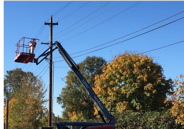
Stay at least 10 feet back from power lines!
